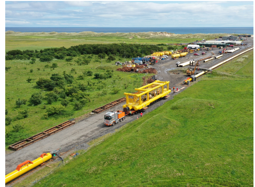
Bundle towhead and pipeline at Wick
